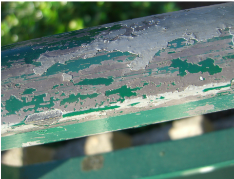
Fig 1 Paint weathered surface
